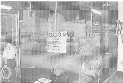
Fig. 2 One of the 200 RT turbo chillers under in-situ measurement
